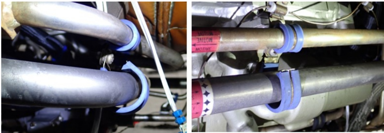
Figure 2. Fractured fuel tube assembly P-clamps
